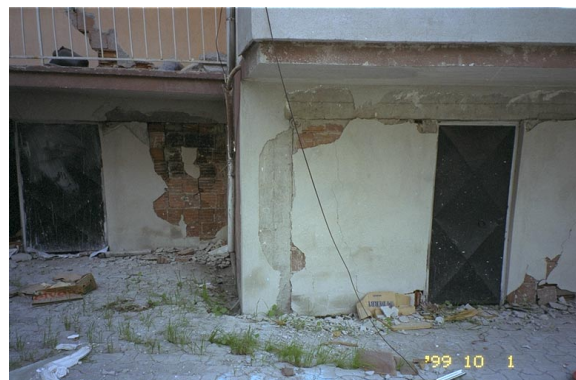
Photo 5.6. Subsidence and damaged infill wall of the building shown in Photo 5.5.
