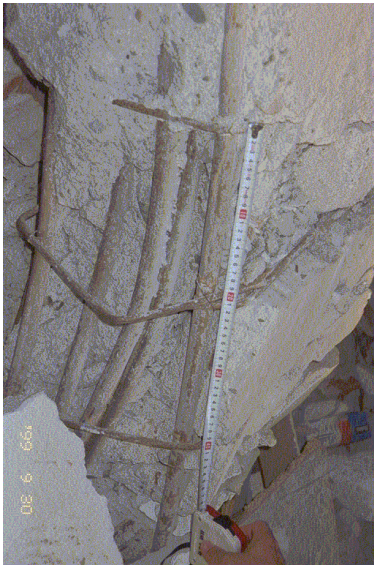
Photo 2.2.7. Reinforcement bar in collapsed column of building, Adapazari.
