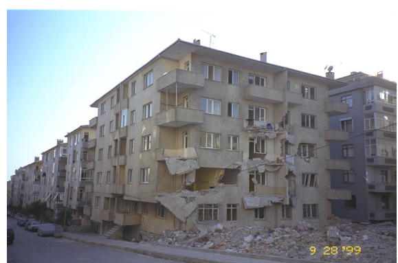
Photo 2.2.16. Residence buildings next to collapsed building in Avcılar.
