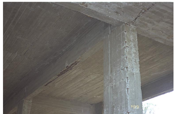
Photo 2.2.10. Exposed reinforcing bars of column and beam, Sapanca.
