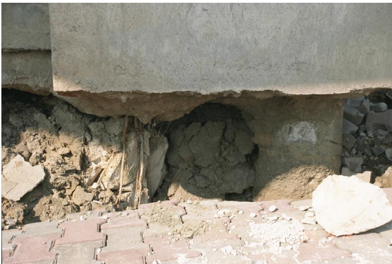
Photo 2.3.3. Damaged pile-head of a gymnasium in Kavakli district, Golcuk, Sep. 1999 (Refer to color Photo 9).
