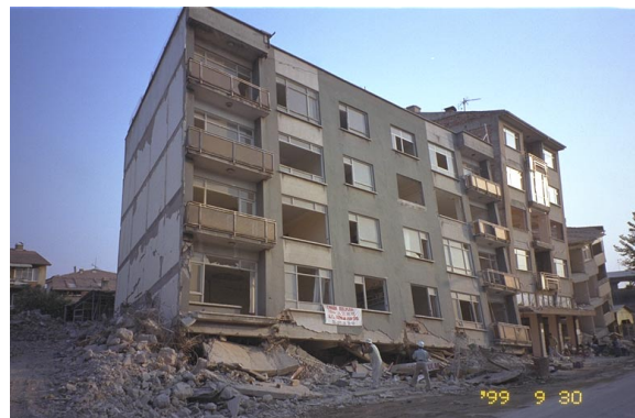
Photo 2.2.2. Residence building collapsed at first story in Adapazari (Refer to color Photo 2).
