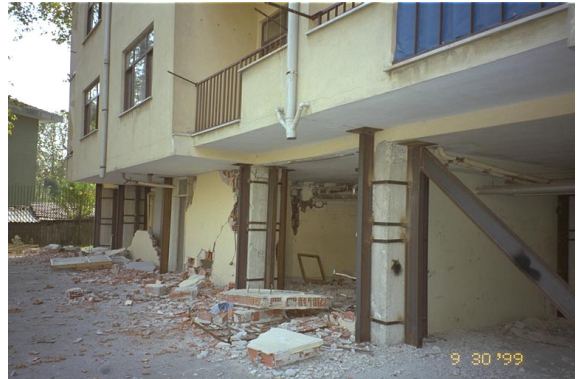
Photo 2.2.14. Damaged columns and walls in piloti of residence building, Yarımca (Refer to color Photo 5).
