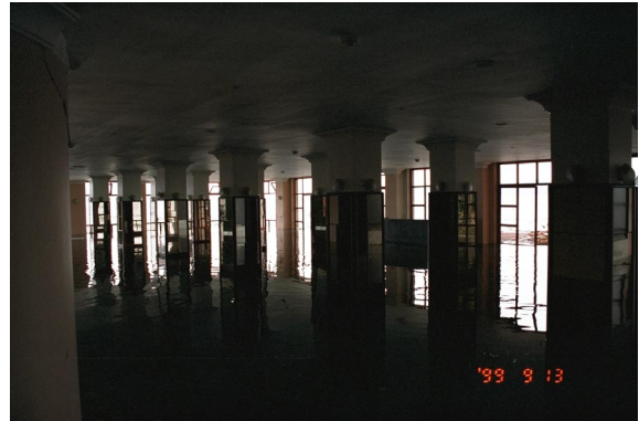
Photo 2.3.7. Submerged 1st floor of Sapanca Hotel, Sep. 1999 (Refer to color Photo 14).
