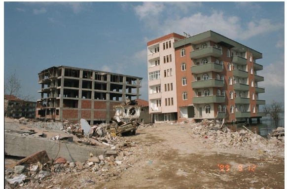
Photo 2.3.4. Depression of ground under buildings in Kavakli, Golcuk, Sep. 1999 (Refer to color Photo 10).
