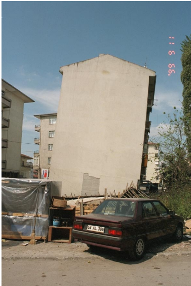
Photo 2.3.12. Inclination of Building B in Adapazari, Sep. 1999.
