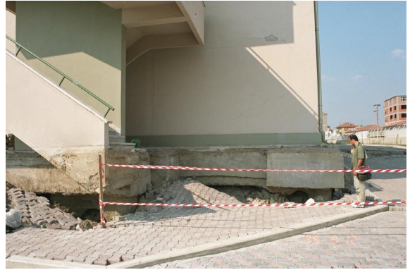
Photo 2.3.2. Exposed pile-foundation of a gymnasium in Kavakli, Golcuk, Sep. 1999 (Refer to color Photo 8).
