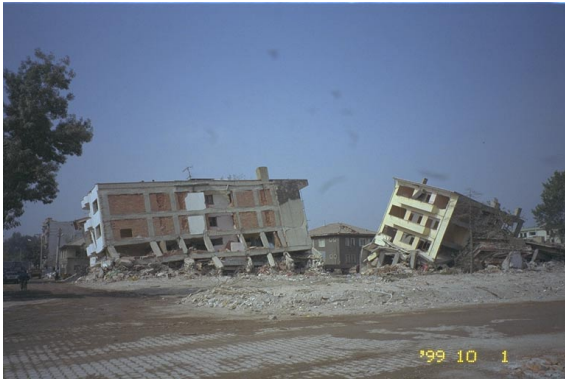
Photo 2.2.13. Collapsed buildings caused by ground failures in Adapazarı (Refer to color Photo 4).
