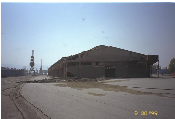
Photo 2.2.15. Warehouse damaged by crane fall, Derince Port.
