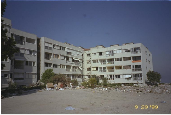
Photo 2.2.11. Collapsed first story of residence building in Aydıncık.
