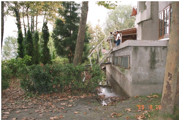
Photo 2.3.8. Relative displacement between ground and building in Sapanca, Sep. 1999 (Refer to color Photo 15).
