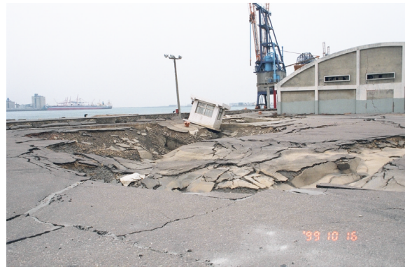
Photo 2.5.2. Ground depressions at North terminal in Taichung Harbor (Refer to color photo 18).
