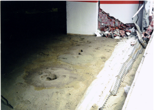
Photo 2.5.7. Remarks of sand boils at basement floor of Building B in Nantou city (Provided by Mr. Hitoshi Kumagai).
