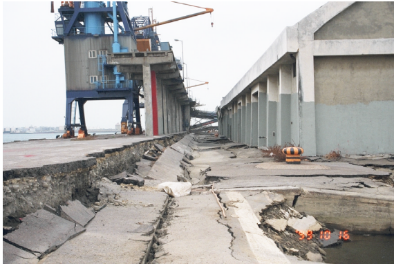
Photo 2.5.1. Settlement of backfills at North terminal in Taichung Harbor.
