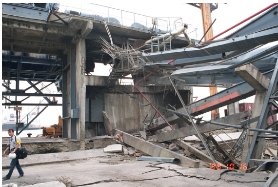
Photo 2.5.3. Collapsed belt conveyer facility at North terminal in Taichung Harbor.
