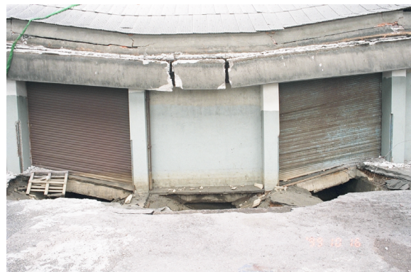
Photo 2.5.4. Collapsed R/C warehouse at North terminal in Taichung Harbor.
