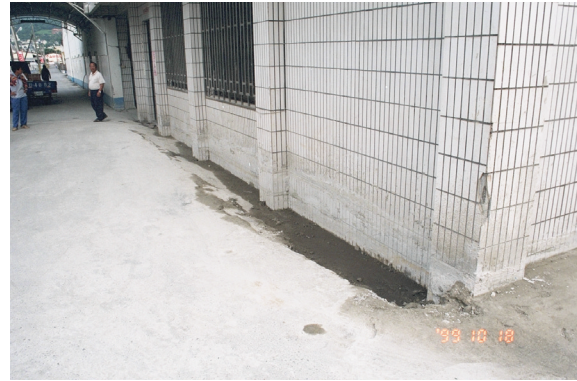
Photo 2.5.9. Settlement of Building E in Yuanlin district.
