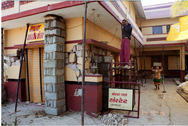
Photo 3. Damage to the buildings (from outside).
